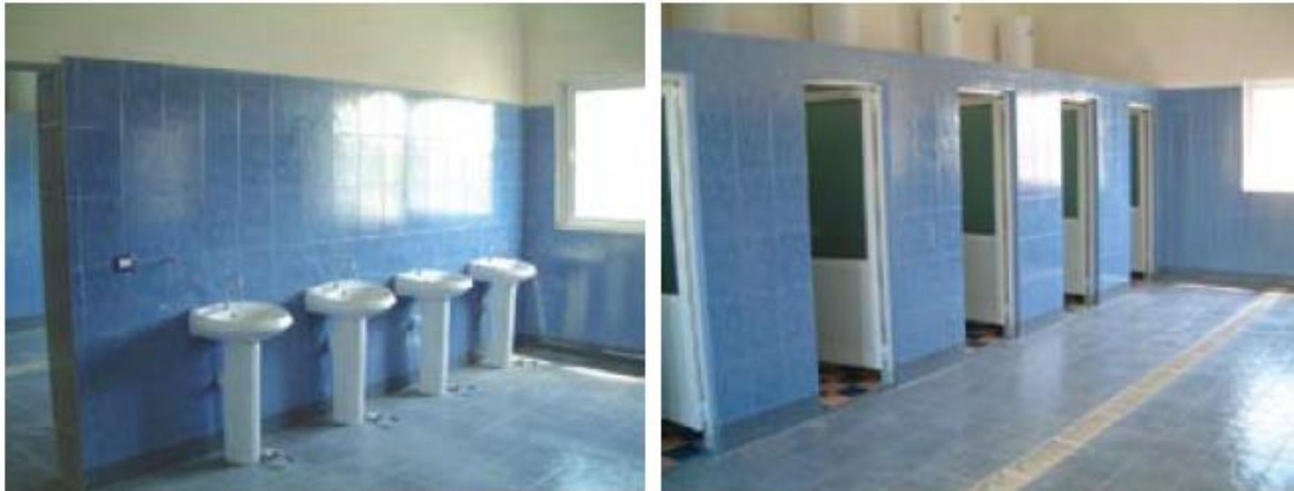
FIGURE 37 Wash-hand basins and showers
