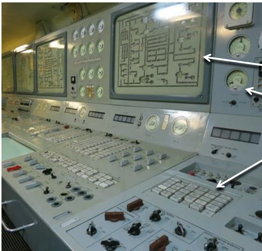
Fig. 15-4 This panel shows many discrete devices as well as mimic panels showing process lines.
