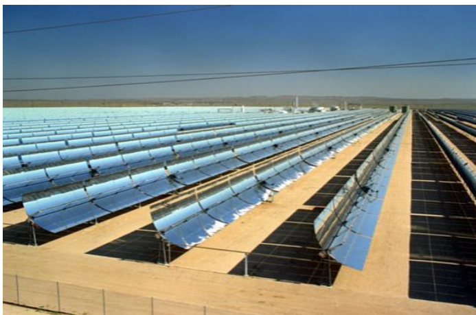
Figure . Parabolic trough system .
